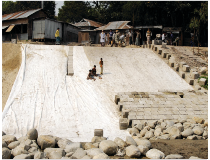
River bank protection activities along the Brahmaputra River, which completely dries up during the dry season and floods over during the rainy season.
